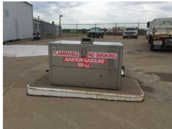
Photo of Existing 100 LL Fuel Cabinet
