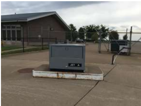
Photo of Existing Jet A Fuel Cabinet
